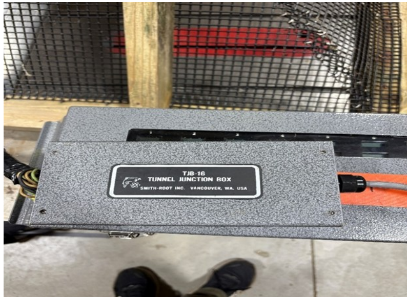
Figure C.2. A view of the cover of the tunnel junction box. Four screws to remove the box cover are located on the top corners.
