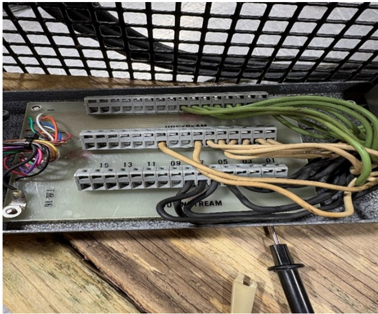
Figure C.6. The white wire on the left side of the middle bar is moved to another terminal to test for failure of the initial terminal.
