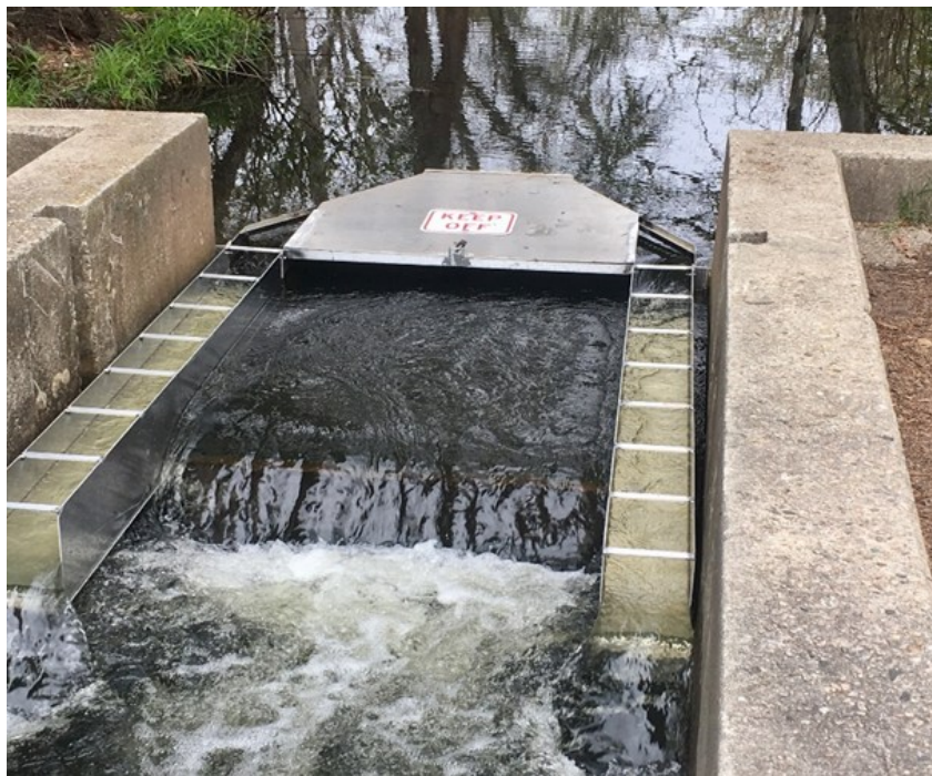
Figure 2.5. Smith-Root 1601 counter with downstream migration chutes installed, Herring River, Harwich.
