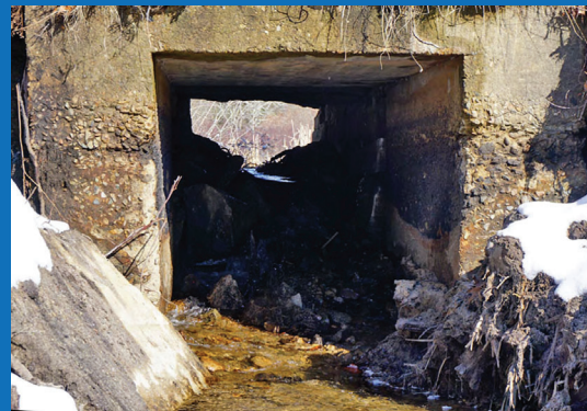
February 2021 – Deteriorated, Blocked Culvert
