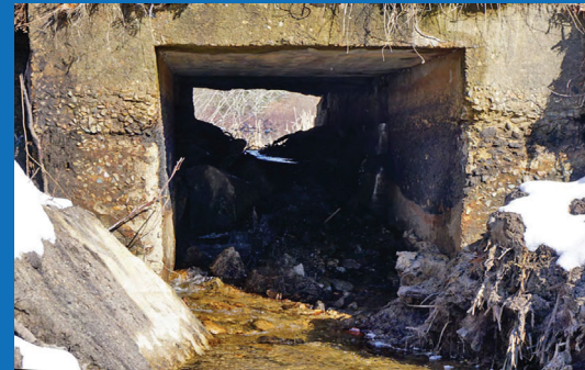
Early February 2021 – Deteriorated Culvert
