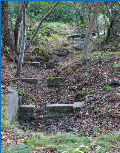
August 2020 Non-functional Fish Ladder
