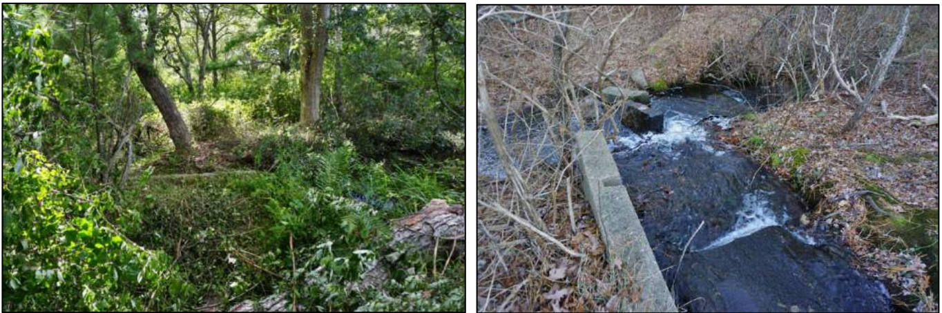
Figure 3: Left: Photo of the earthen berm or dam (credit: Falmouth Rod and Gun Club). Right: Photo of the spillway with concrete pieces broken away from the structure (credit: Falmouth Rod and Gun Club).
