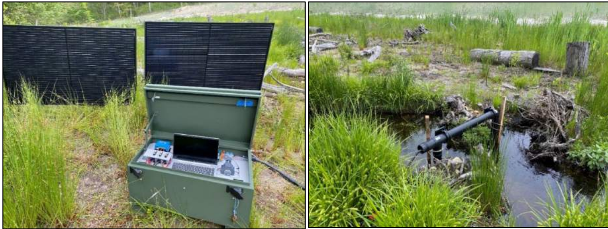
Figure 12: New antenna reader and solar panels ( left ) along with PIT antenna ( right ) installed on May 31, 2022, in the former pond area near the Falmouth Rod and Gun Club along with laptop for download. PIT-tagged Brook Trout are detected when they swim through the antenna (credit: Steve Hurley).
