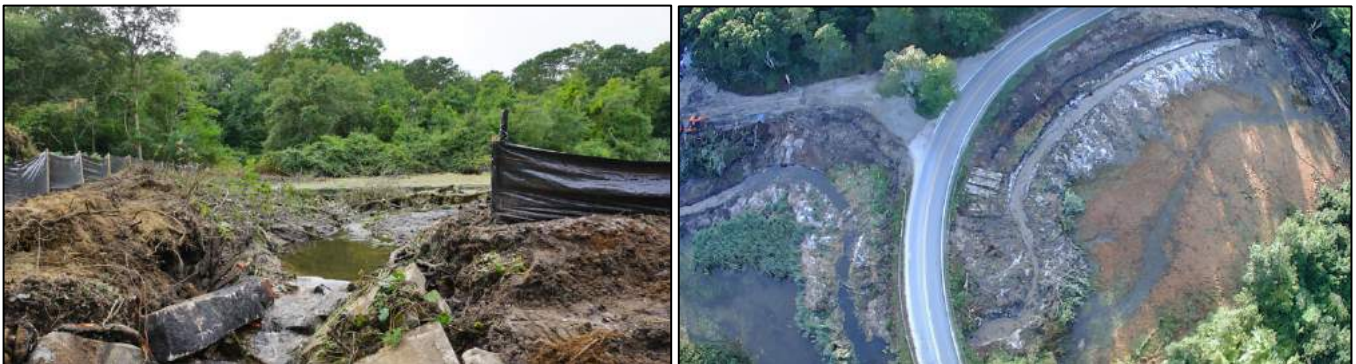
Figure 5: Left : Photo of dam spillway removal (credit: Falmouth Rod and Gun Club). Right : Aerial of diversion channels created north and south of Carriage Shop Road (credit: Falmouth Rod and Gun Club.).
