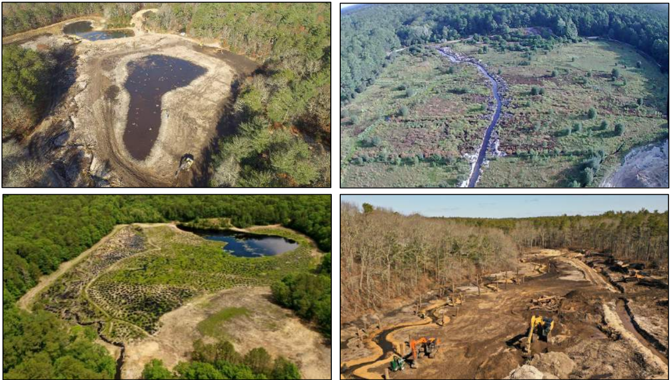
Figure 6: Top left: Creation of new stream channel and shallow ponds in the former Garner Pond, fall/winter 2020-2021 (credit: Inter-Fluve, Inc.). Top right: Diversion channel created in Farley Bog prior to regrading and new channel, October 2020 (credit: Falmouth Rod & Gun Club). Lower left: Completed construction and early revegetation of Farley Bog in spring 2021 (credit: Inter-Fluve, Inc.). Bottom right: Removal of impoundment north of Carriage Shop Road and creation of the new river channel (credit: Inter-Fluve, Inc.).
