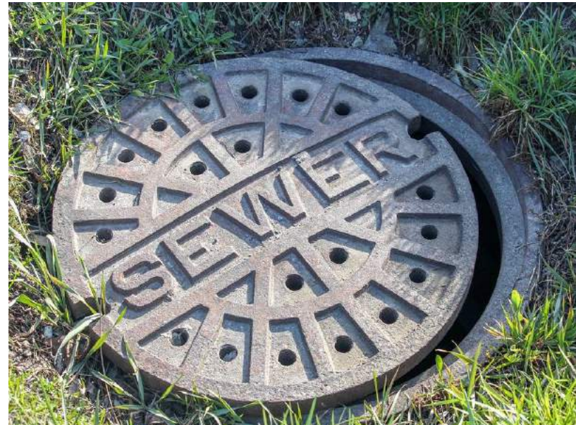
Figure 30. Sewer manhole cover (Pixabay).
