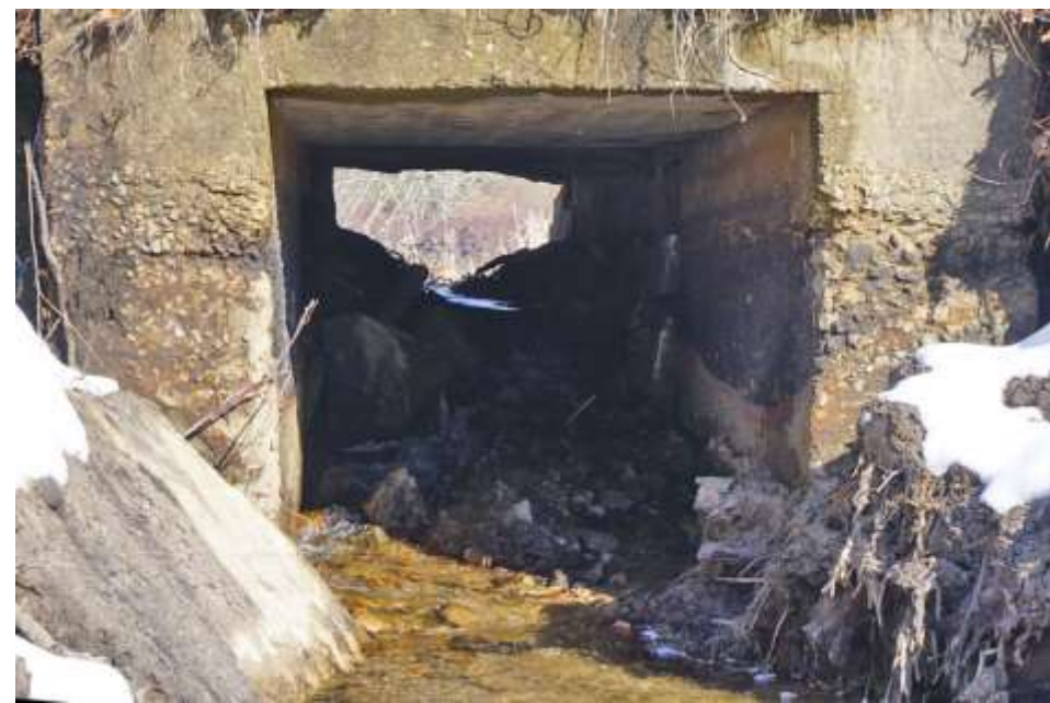
Clogged / Deteriorated Culvert
