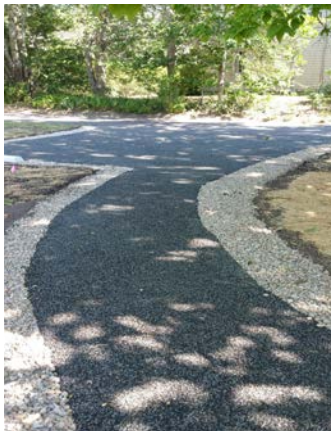
APCC believes that this may be the first installation of Porous Pave® for parking and path on the Cape.
