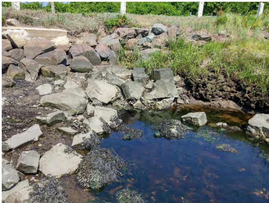
Photo 9. The impaired Stage Harbor Road culvert (Chatham, MA) is buried under a pile of rocks on the seaward side of the marsh.
