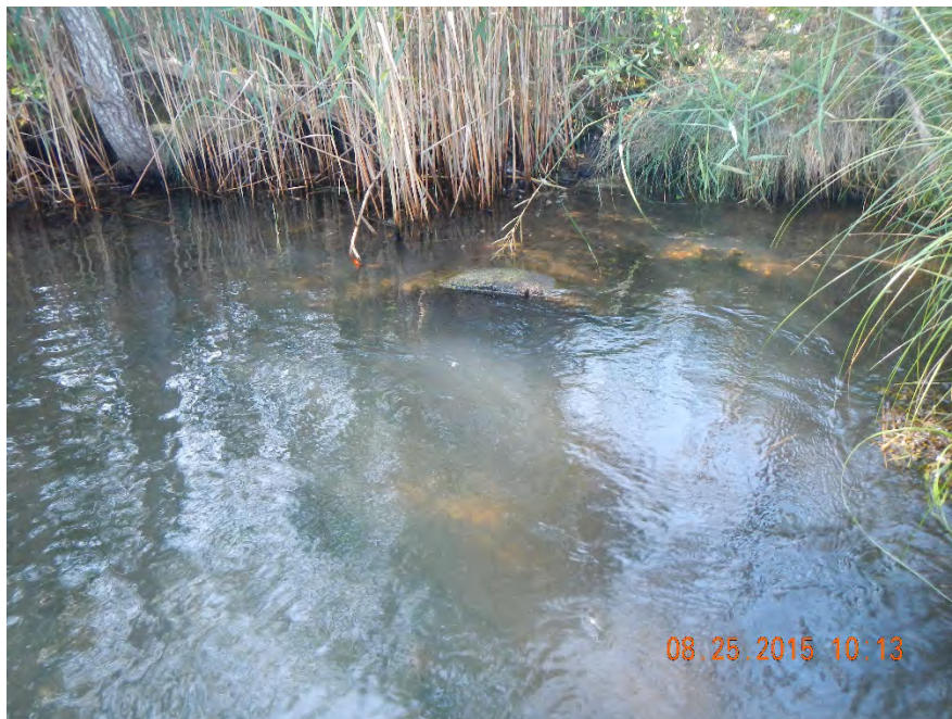
Photo 11. Flooded culvert at Weir Creek salt marsh during high tide.
