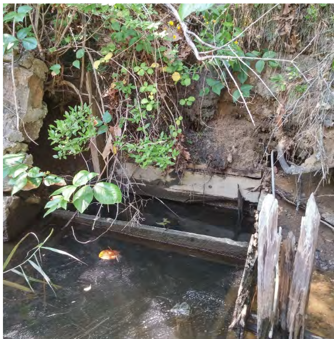
Photo 1. Culvert that is limiting tidal flow into an unnamed salt marsh (BN-39) on Little Buttermilk Bay in Bourne, MA. This image is taken from the restricted side of the marsh and the metal culvert appears to be covered with slumping earth and rotting boards.
