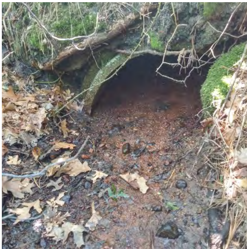
Photo 3. Small culvert filling with sediment between located between BN-39 salt marsh and Barrows Bog (Bourne, MA).
